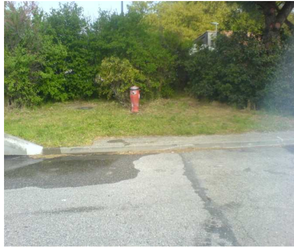
Poteau incendie aire ouest-sud station service
